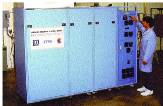
Testing of the 25kW power system.
